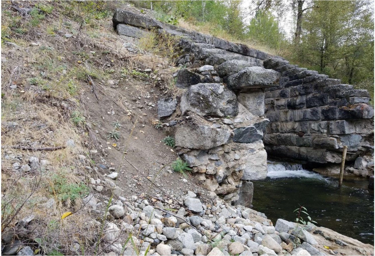
Outlet wingwall failure and sloughing
