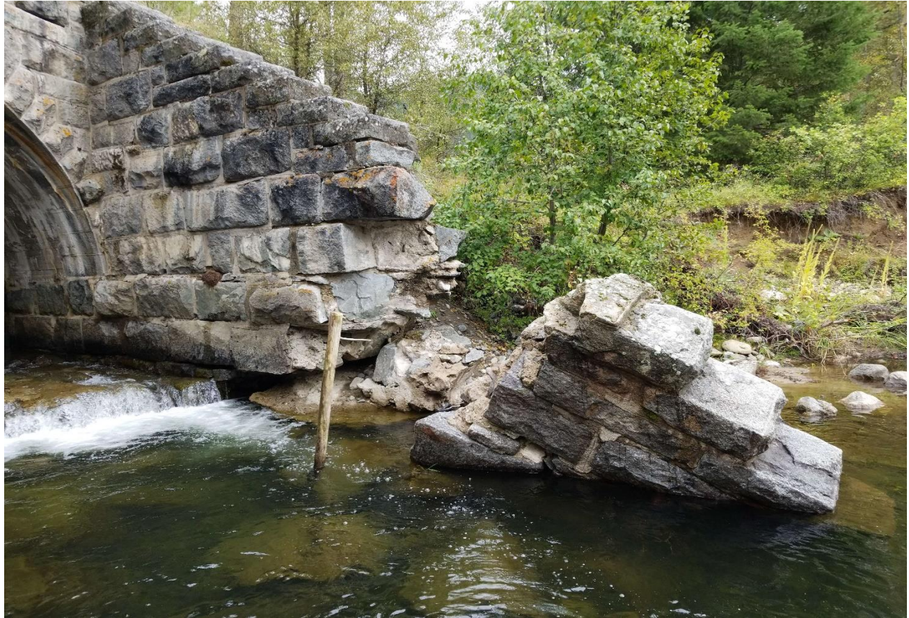
Outlet wingwall failure
